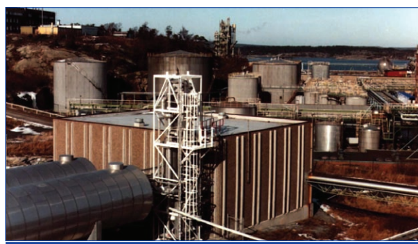
Figure 5. Costain designed carbon dioxide liquefaction plant for the food industry.
